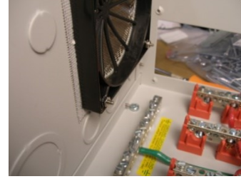
E-Panel earth ground bus (AC & DC)
